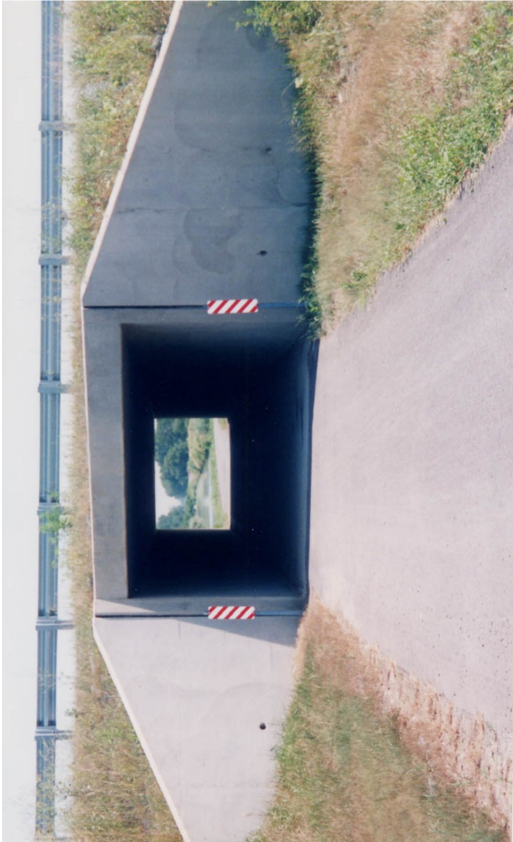
BOX COLVERT INTENDED FOR FUTURE BIKEWAY
